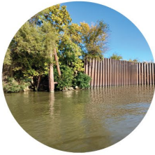
SEA WALL CONDITION
